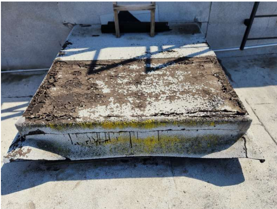
Lower North Roof Air Vent next to wall dividing Upper and Lower Roofs
